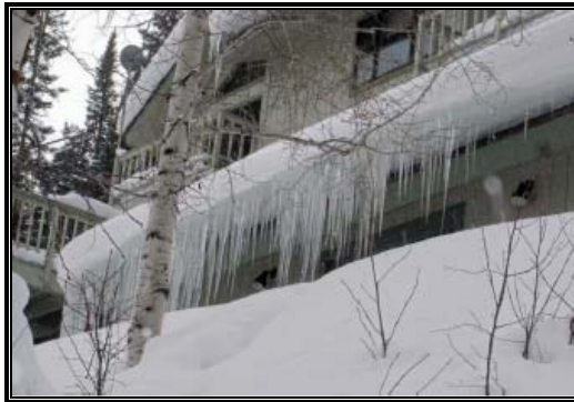
Heavy Ice Damming at Roof's Edge
