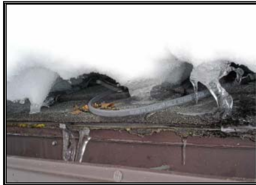
Roof Mounted Heat Tape
